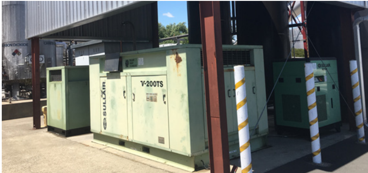
One winery relies on multiple Sullair stationary compressors for its operation
